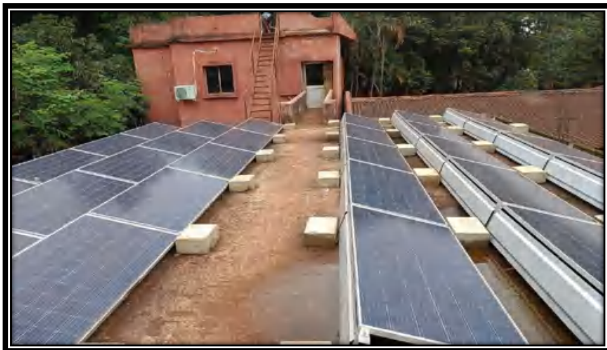
PHOTOGRAPH SHOWING 30KVA SOLAR POWER
